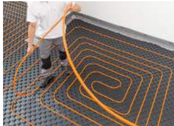
Hot water under-floor heating
